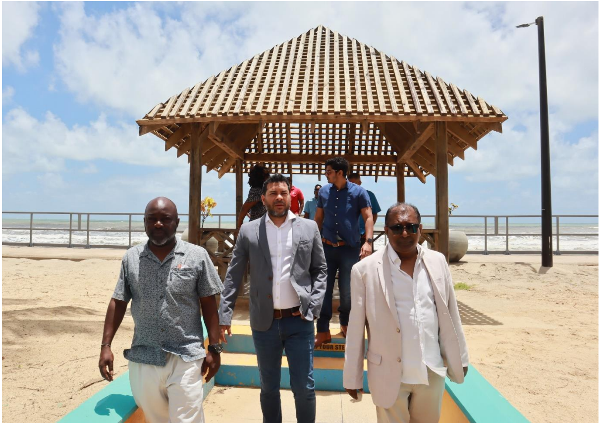
Minister of Tourism, Culture and the Arts, Senator the Honourable Randall Mitchell and Member of Parliament for Cumuto/Manzanilla, Dr. Rai Ragbir, are brought up to speed on the Manzanilla Beach Facility refurbishment works by members of the Ministry's Projects and Facility Management team.
